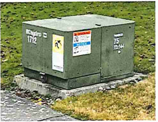
Pad Mount Transformer (PMT)
